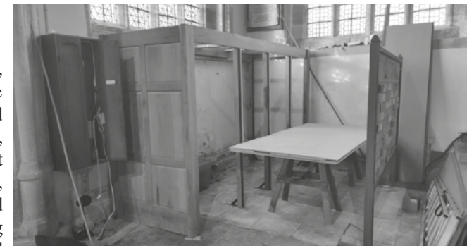
Construction of the new cabinet for the chairs in St Mary's Church
